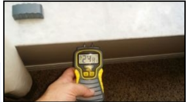
Elevated moisture levels below master bedroom window
