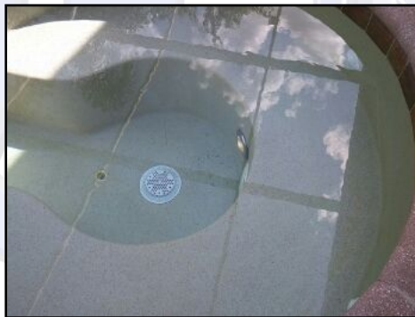
Spa light functioning
