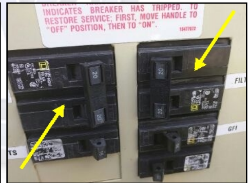
Recommend GFCI on pool pumps, heater
