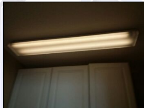
Ballast low in fluorescent
