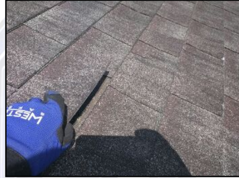
Seal strips loose
