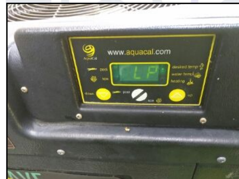
Pool Heater inoperable
