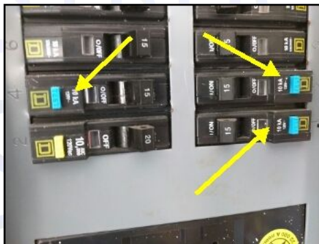
Recalled breakers blue test button
