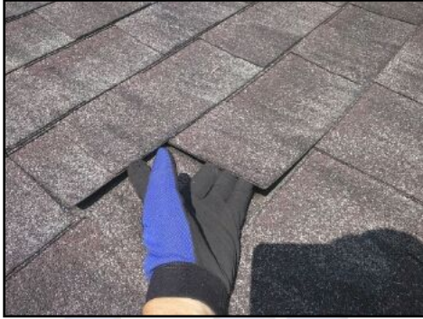
Seal strips loose
