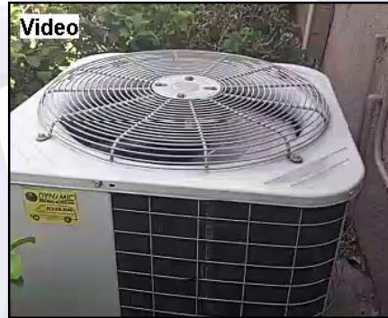
Video: Condenser Operating
