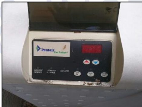
Spa heater inoperable
